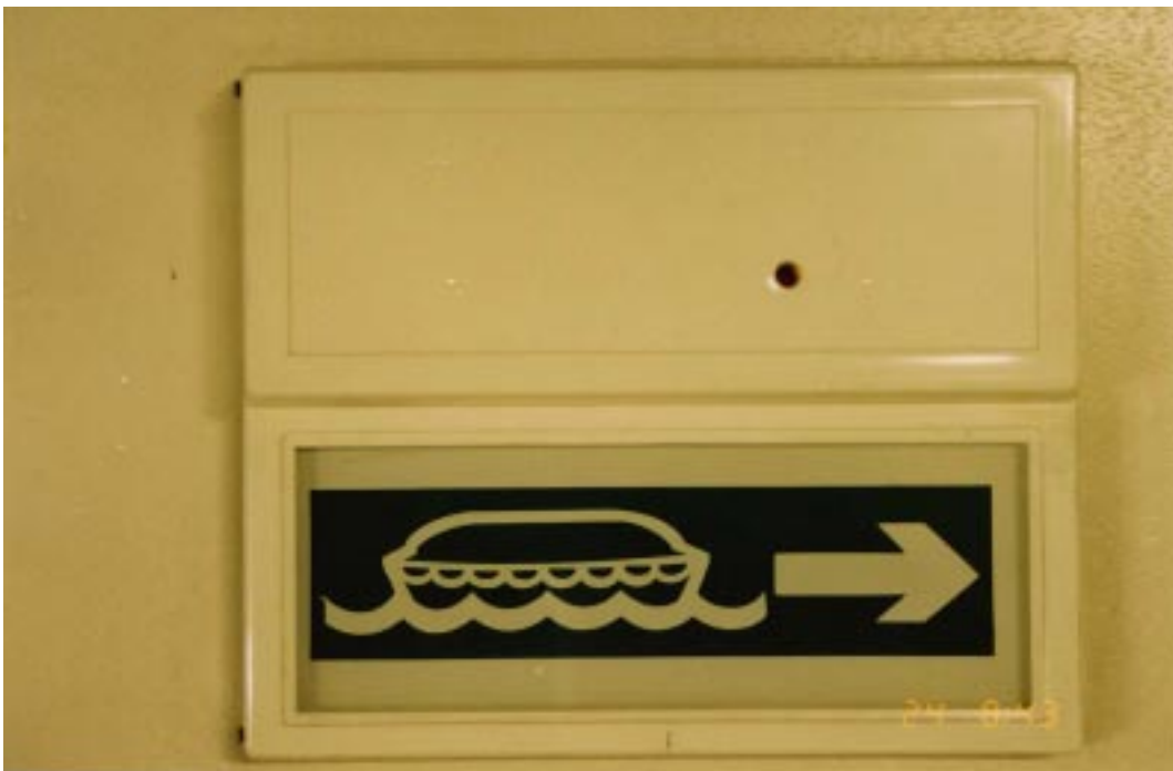
b) fluorescent lamp operated signal light.
